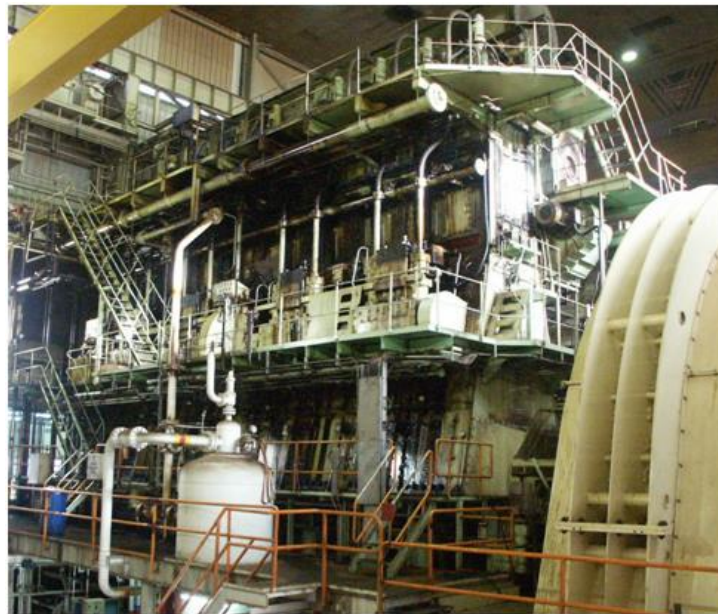
Fig.28. A nine-cylinder Sulzer RTA76 diesel engine producing 25 MW of power at 95 rpm.
