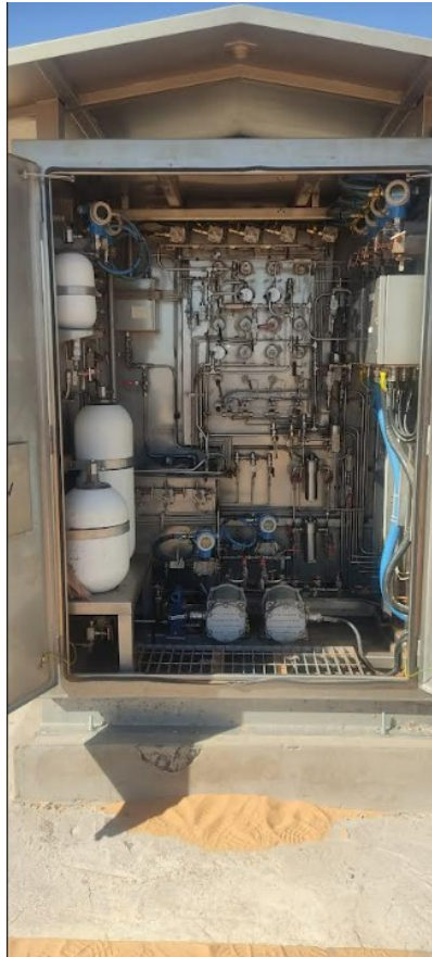
Figure 1.11: Wellhead Control Panel(WHCP)
