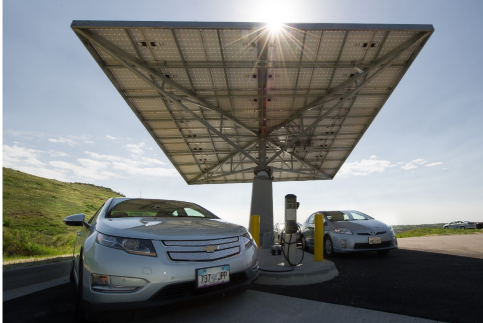
Figure 1.6: Appearance of new charging systems for EV's
