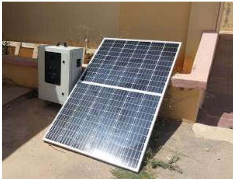
Figure IV-10: Photographs of the installed system.
