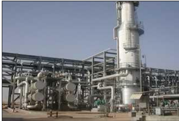
Fig 1.6: HP stabilization section [photo taken during the training]
