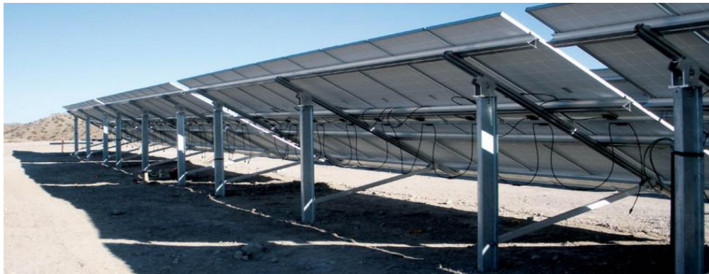
Figure 2.14:le champ photovoltaïque.
